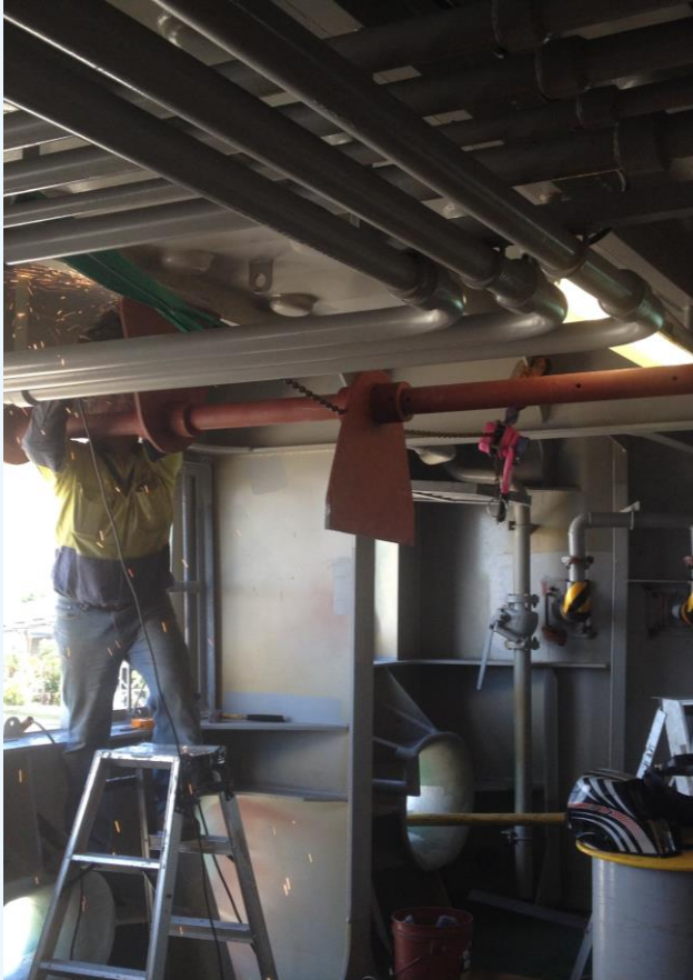
Above: Welder from Stella Marine Group (Brisbane) attaching the ‘push out tow point’ on the Salome .
