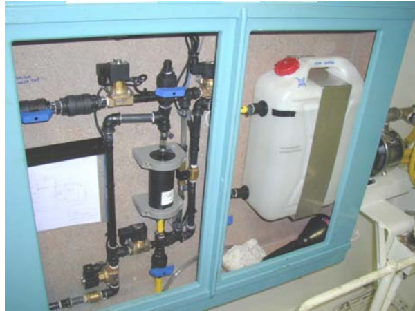
Fig. 2. Sampling manifold in engine room of SOOP vessel used in the COOE project. A present-day system could be more compact and potentially relocatable than that depicted.
